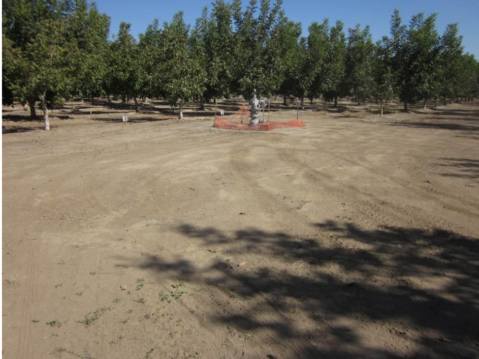
Photo 3: Well conversion activities have been completed at the Southam #2 well site. All equipment has been removed and final grading completed.
