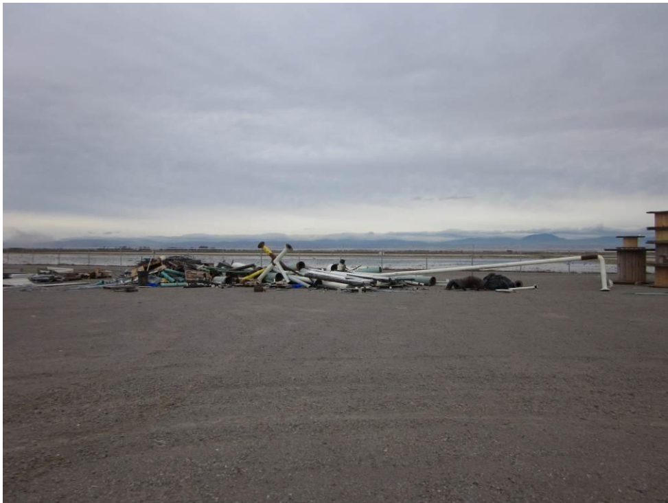
Photo 4: Construction-related materials remain in the northern portion of the Compressor Station site.
