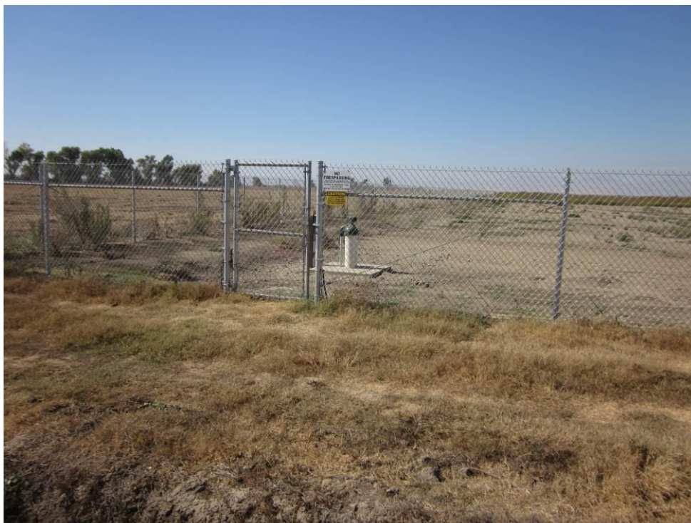
Photo 1: Two cathodic protection wells have been installed in the 5-acre buffer area surrounding the temporary compressor at the Remote Well Pad site. Pictured is the completed well in the southeast corner of the site.
