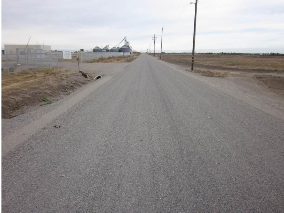
Photo 5: Final repairs and paving of McAusland Road, Southam Road, and Dodge Road were underway. Pictured is completed paving along McAusland Road.
